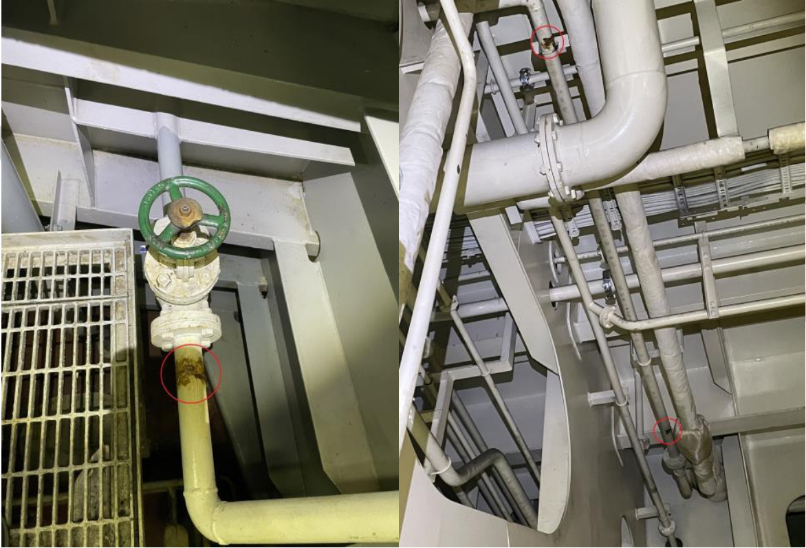
Pictures of other deficiency: Cooling seawater outlet for deck machinery found leaking in 3 locations
